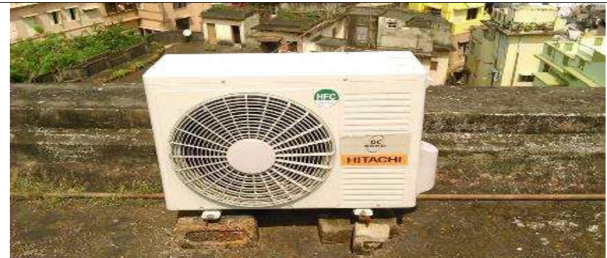
Use of new generation Air conditions with HFC R401A coolant
