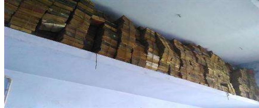
Exhibit 6 - Old stock of unused books inside classroom thereby increasing fire load
