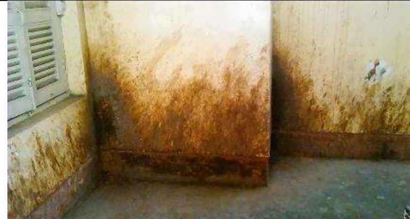
Exhibit 2 - Unhygienic condition in common student room
