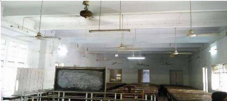
Exhibit 3 - Energy loss (Fan & lights running in empty room)
