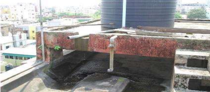
Exhibit 5 - Roof top water tank overflow spillage
